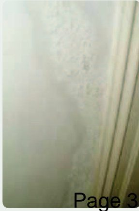
Rising damp is affecting the paint finish causing it to bubble.
